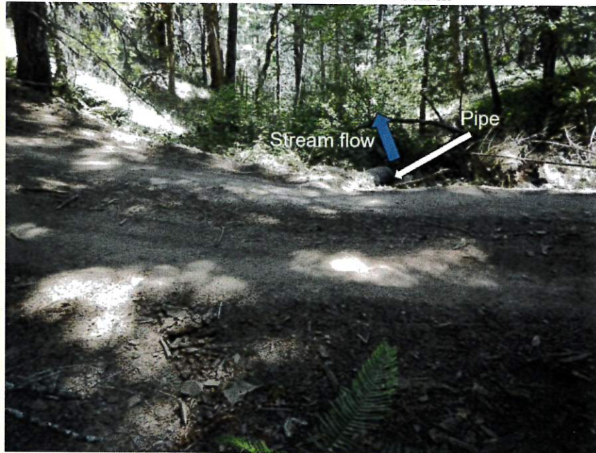
Figure 1—Photo looking downstream at the road crossing an unnamed tributary to the Mad River on the Szagora LLC property. The existing culvert is too small and does not meet industry sizing standards. Thus, when the stream is running full, water can flood the road and carry road material and fine sediment back into the waterways. Fine sediment can make it difficult for fish to breathe, find food and refuge, and reproduce.
