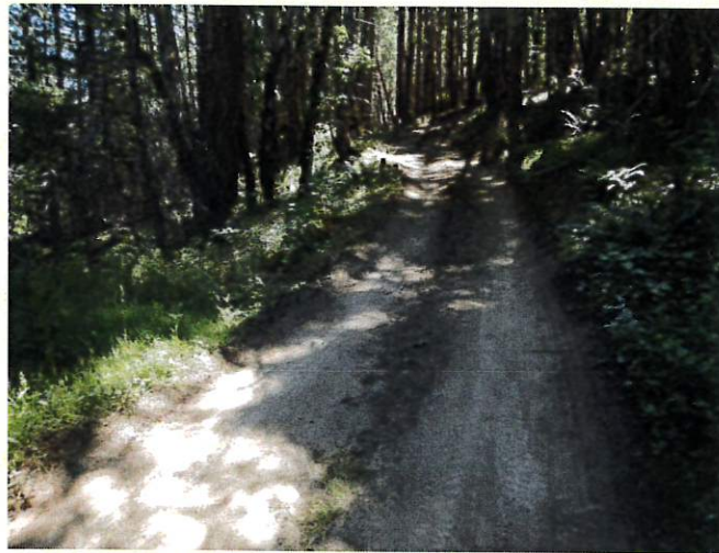
Figure 2— Looking east along a dirt road approaching a stream crossing on the Szagora LLC property. The road is steep and lacks key features, such as water bars or rolling dips, to direct stormwater off the road and minimize sediment delivery to the stream. This leaves the road's earthen surface susceptible to erosion by stormwater, which is likely to carry excess fine sediment from the road into the stream.
