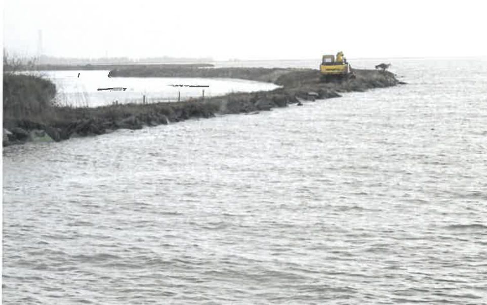
LEVEE PROTECTION: Humboldt Bay crept up the levees during a recent record high tide. The water behind this levee just east of the Mad River Slough is from rainfall. Photo: Jack Durham | Union
