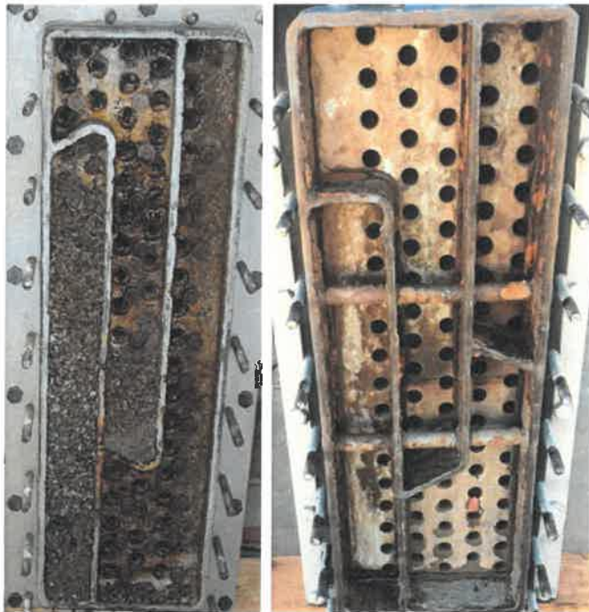
1. A Parker Dam heat exchanger that was pulled for maintenance before the Hydro-Optic ultraviolet (HOD UV) treatment implementation (left), and the same unit, exposed for the same time and similar conditions, after treatment with HOD UV (right). Courtesy: Parker Dam staff/Bureau of Reclamation
