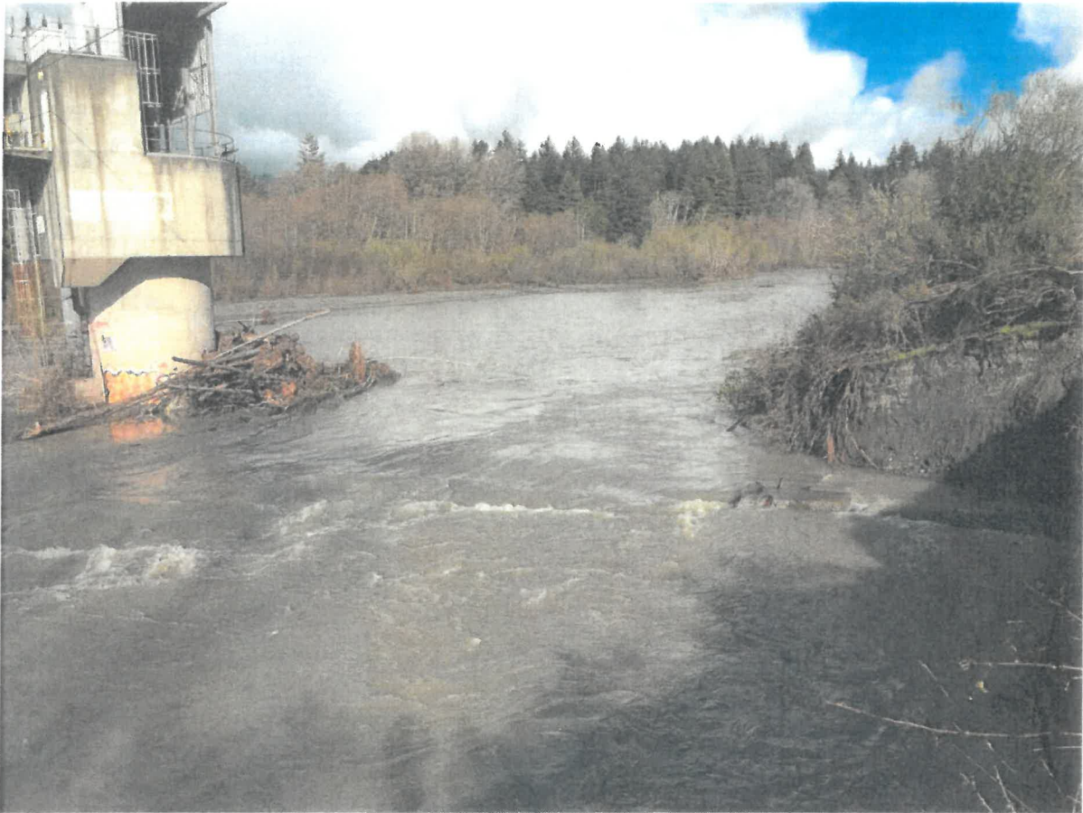
Bank around pipe erosion, looking toward Collector 4 (March 2019)
