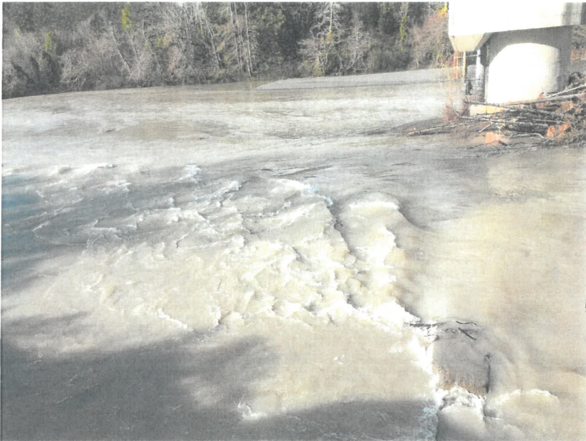
Photo 4 Exposed pipe from Collector 4 (March 2019)
