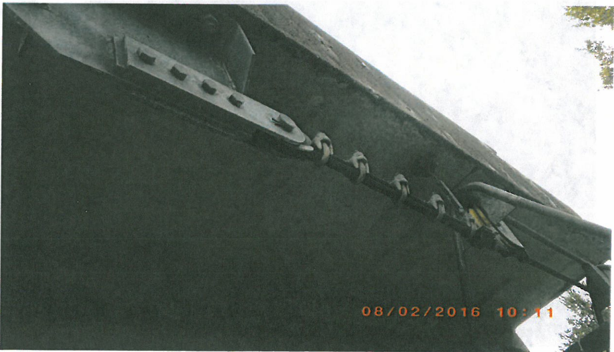
Photo 8 – Trolley #2 Cable Connection at Collector Well
