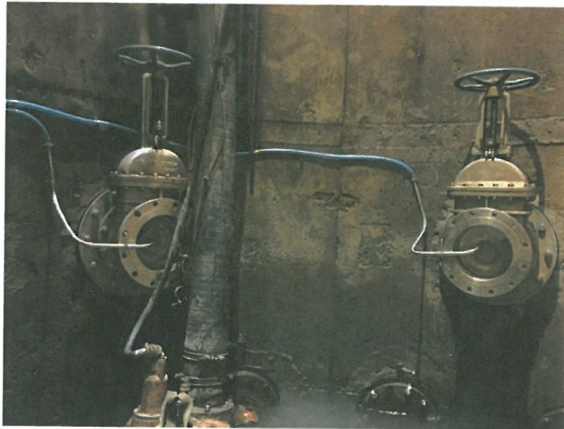
Lateral Valves, Collector 1
