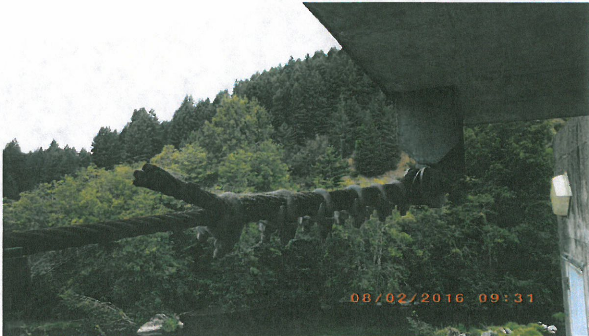
Photo 6 – Trolley #1 Cable Connection at Collector Well
