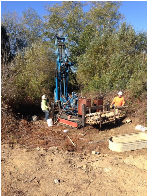
Picture 12: Drill rig being set up at B1 on old railroad grade just off of parking area at NW end of property at 1220 Glendale Drive, McKinleyville, CA.
