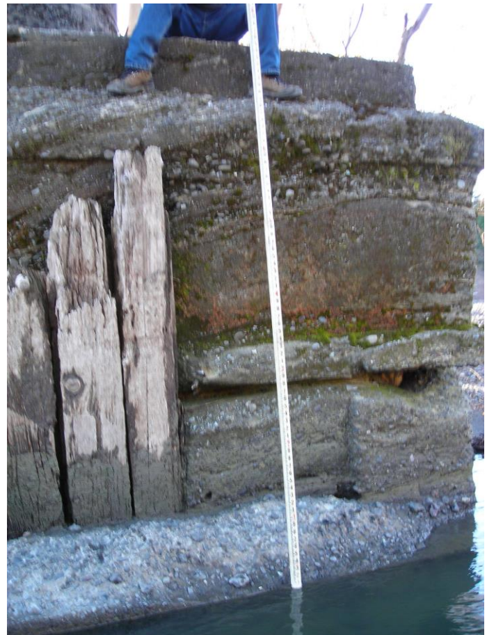
FOOTING PIER 3 FROM RIVER. NOTE ROD SHOWING PIER AND WATER DEPTH AND EXPOSED PILE AT PIER CORNER.
