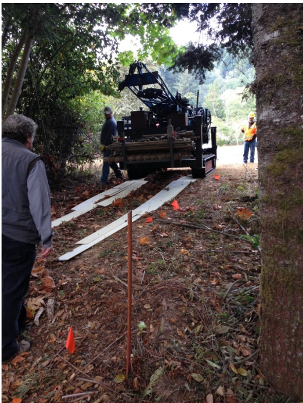
Picture 3: Mobilization of the drill rig across archeological site prior to drilling using particle board as mats.
