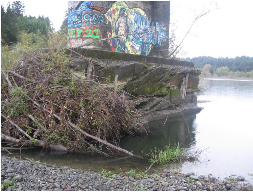
FOOTING PIER 3 WEST SIDE SHOWING EROSION OF TREMMI POURED CONCRETE
