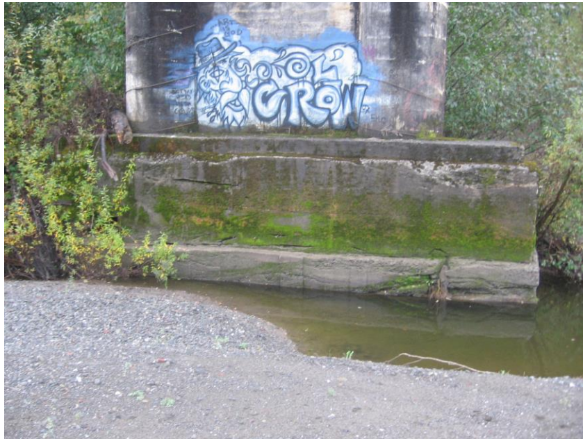
FOOTING PIER 3 FROM UPSTREAM LOOKING AT SCOUR POOL IN RIVER CHANNEL
