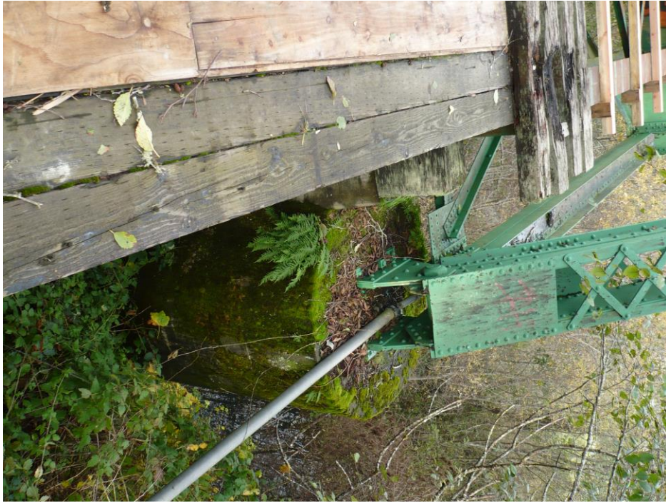
FOOTING PIER 2 AT SCOUR POOL
