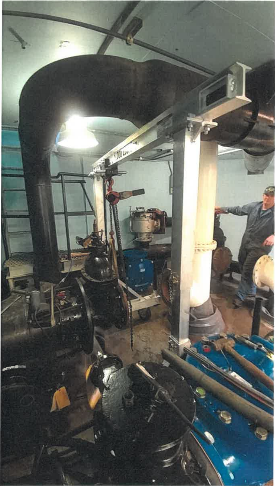
Replacing pump station isolation gate valves and check valves with limited space.
