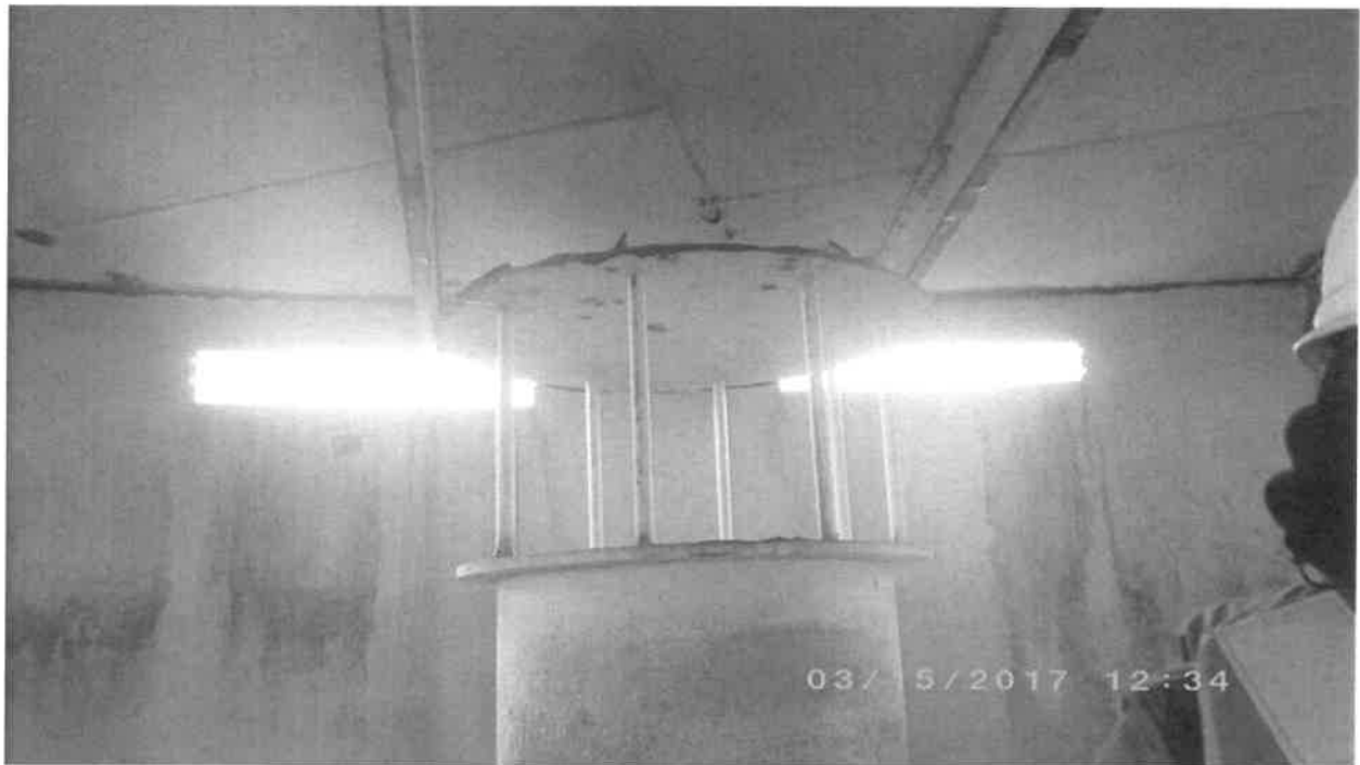
Photo 8 – Over-flow Drain Corrosion
