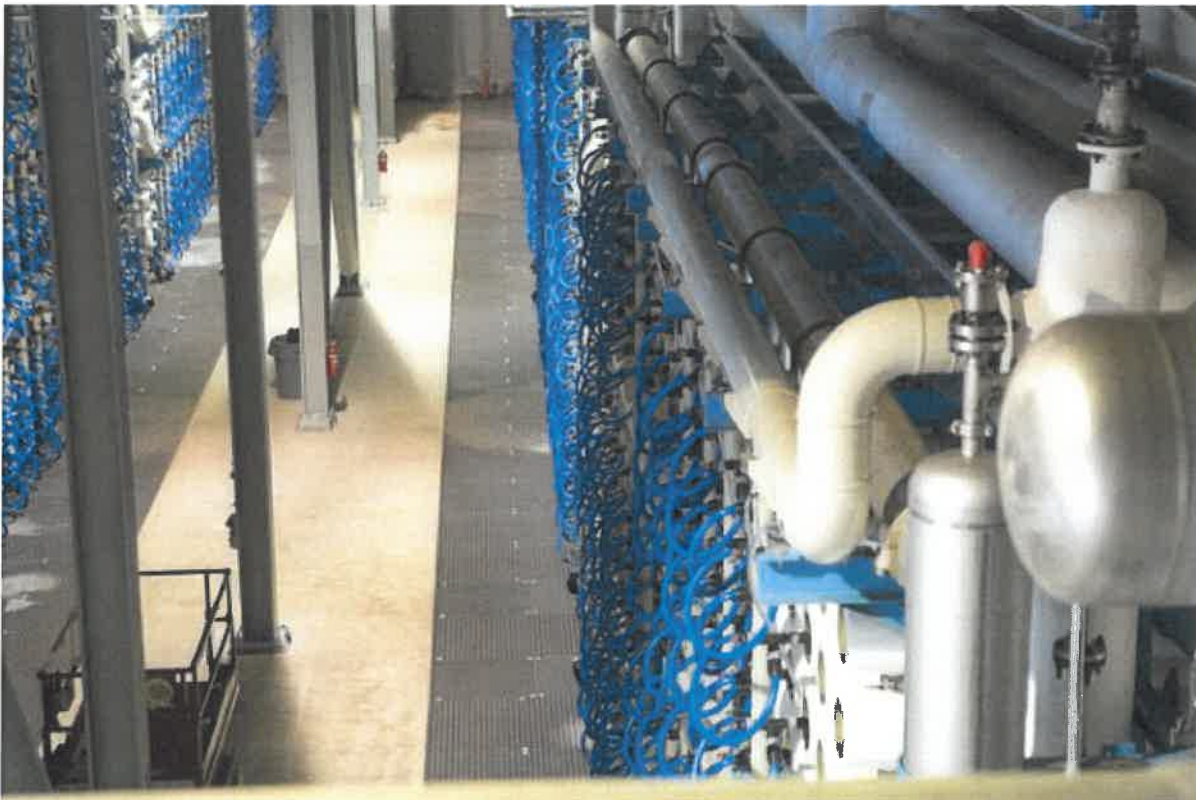
Desalination plant, Carlsbad, Calif. Photo: San Diego County Water Authority.
