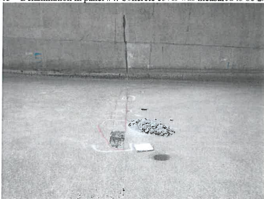
Photo #14 – Delamination in panel #5. Delamination was approximately 50 square feet.
