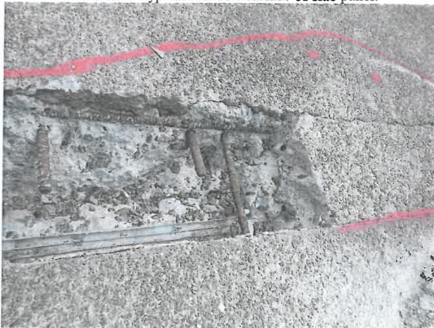
Photo #4 – Section of delaminated concrete removed to expose reinforcing steel at intersection of panels 4 and 5.
