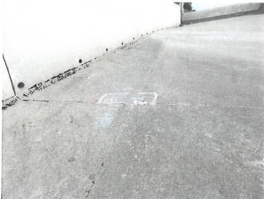
Photo #13 – Delamination in panel #4. Concrete cover was measured to be 2.5 inches.
