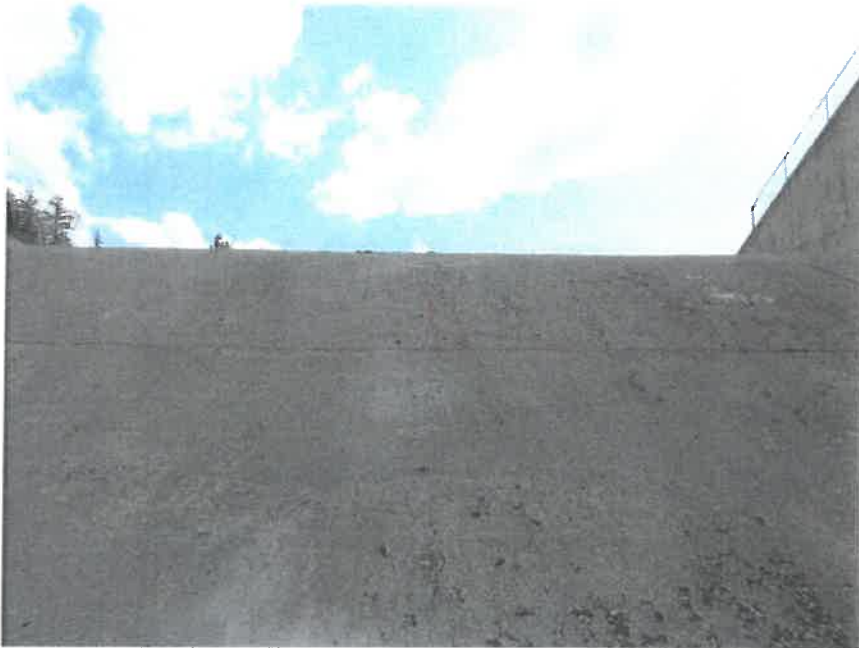
Photo #9 – Delaminated area on Ogee on downstream face near middle.
