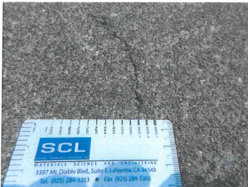
Photo #7 – Typical concrete crack width of 0.040 inches on panel #2.
