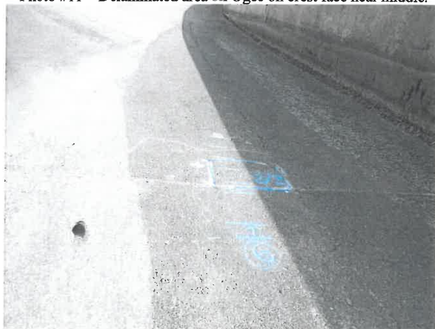
Photo #12 – Delaminated area on panel #3 near panel #2.
