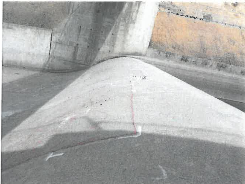
Photo #11 – Delaminated area on Ogee on crest face near middle.
