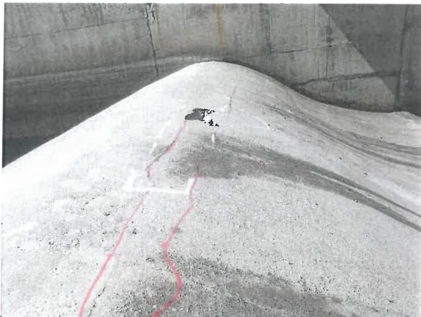
Photo #1 – General view of Ogee crest. Slight scaling of 1/8 inch on surface of concrete.
