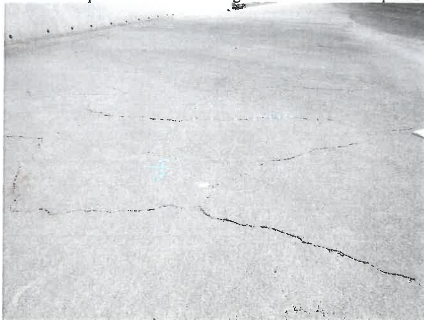
Photo #6 – Concrete cracking pattern in panel #2.
