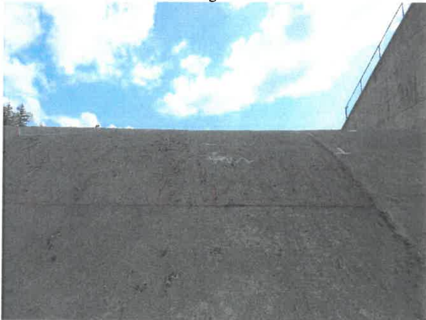
Photo #10 – Delaminated area on Ogee on downstream face near downhill wall.
