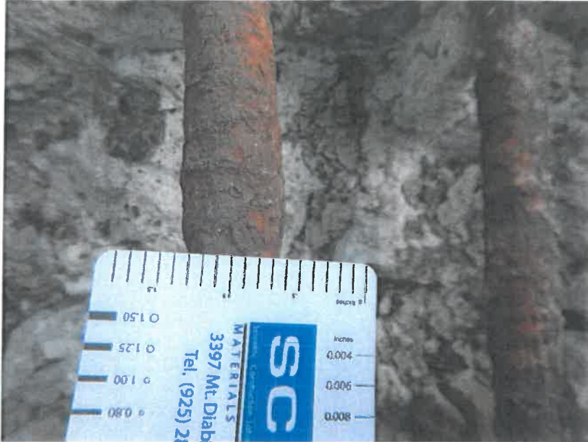
Photo #5 – Close-up of corroded reinforcing steel at intersection of panels 4 & 5.
