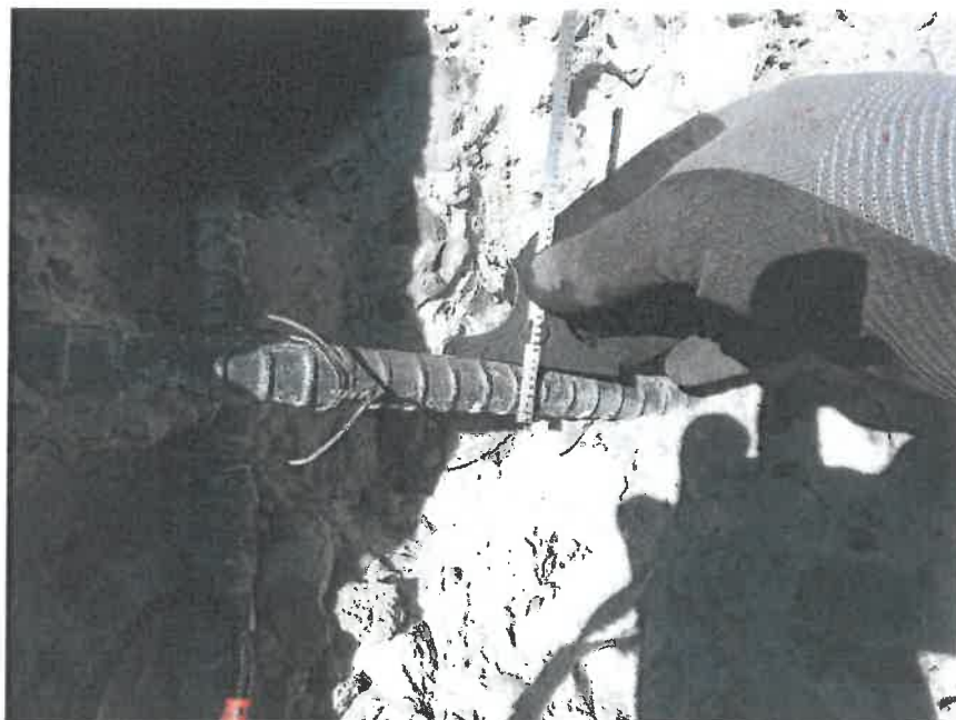
Photo #2 – Exposed reinforcement on Ogee crest.
