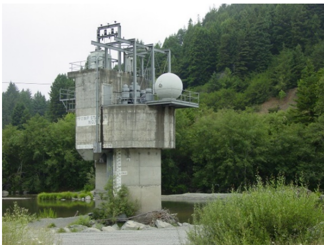
Figure 3. Ranney Well along Mad River, close-up.
