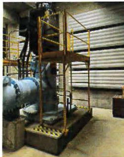
Above: Helix Water District's scaffold system for pump maintenance
