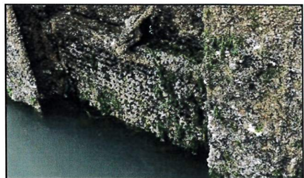
Image 2-16 RMT II-Existing Water Intake Screen
