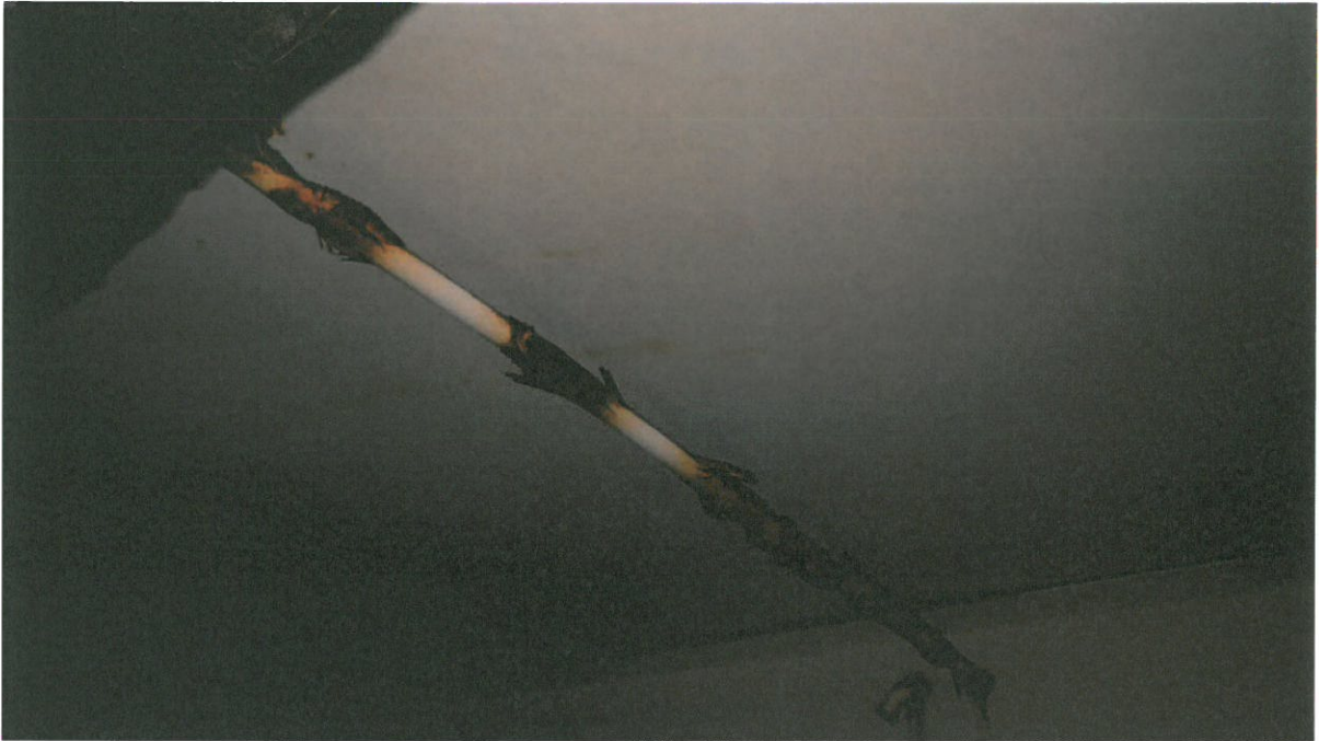
Photo 7 – Rafter Rod Bridging Corrosion
