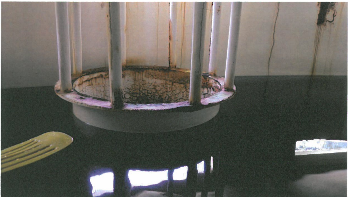
Photo 8 – Over-flow Drain Corrosion
