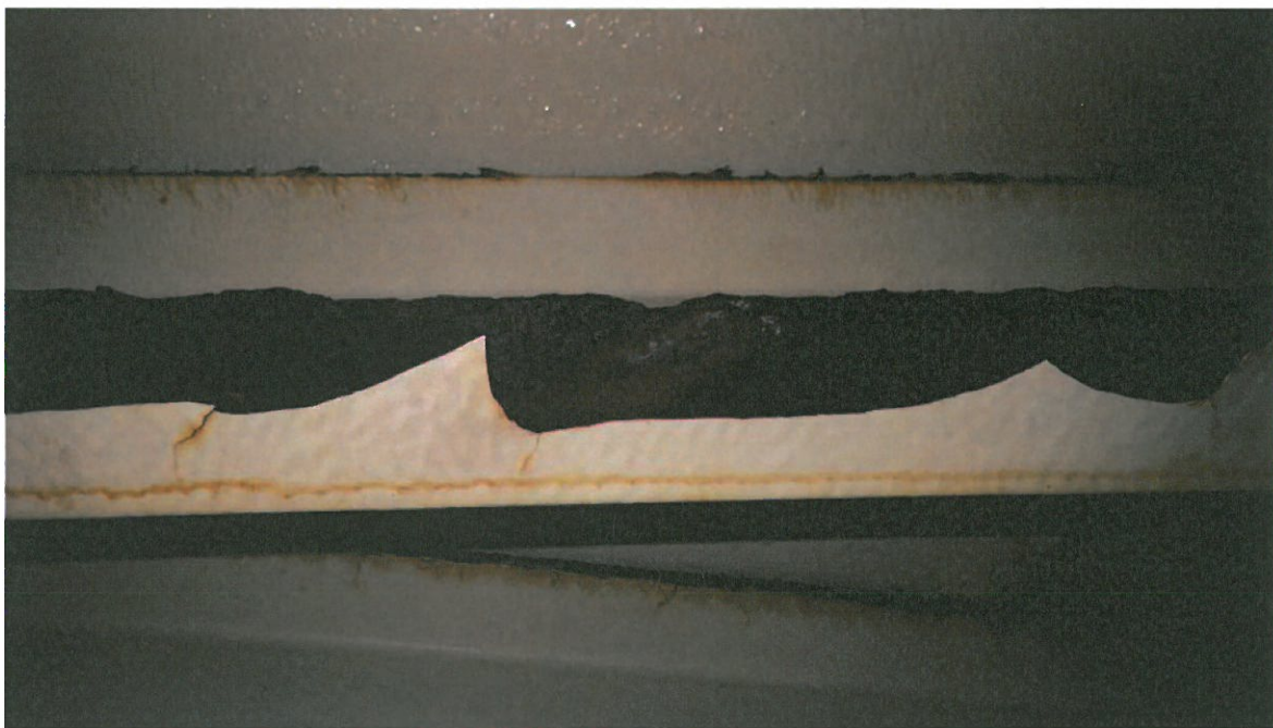
Photo 2 – Material Loss at Channel Bottom Flange
