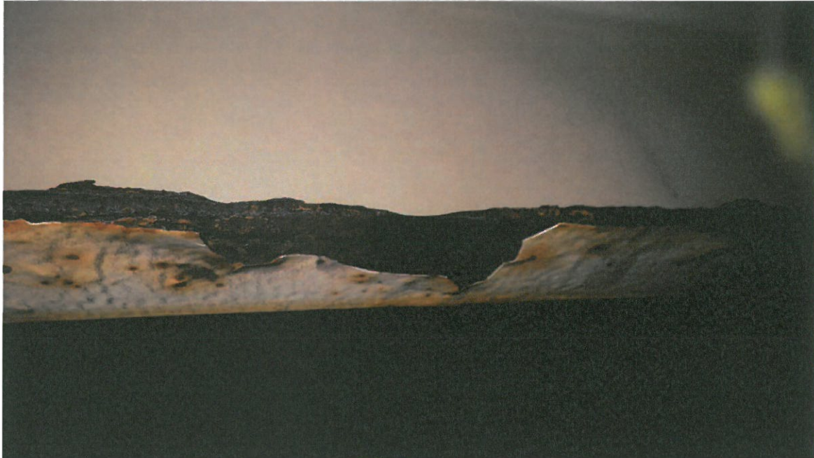
Photo 1 – Material Loss at Channel Bottom Flange
