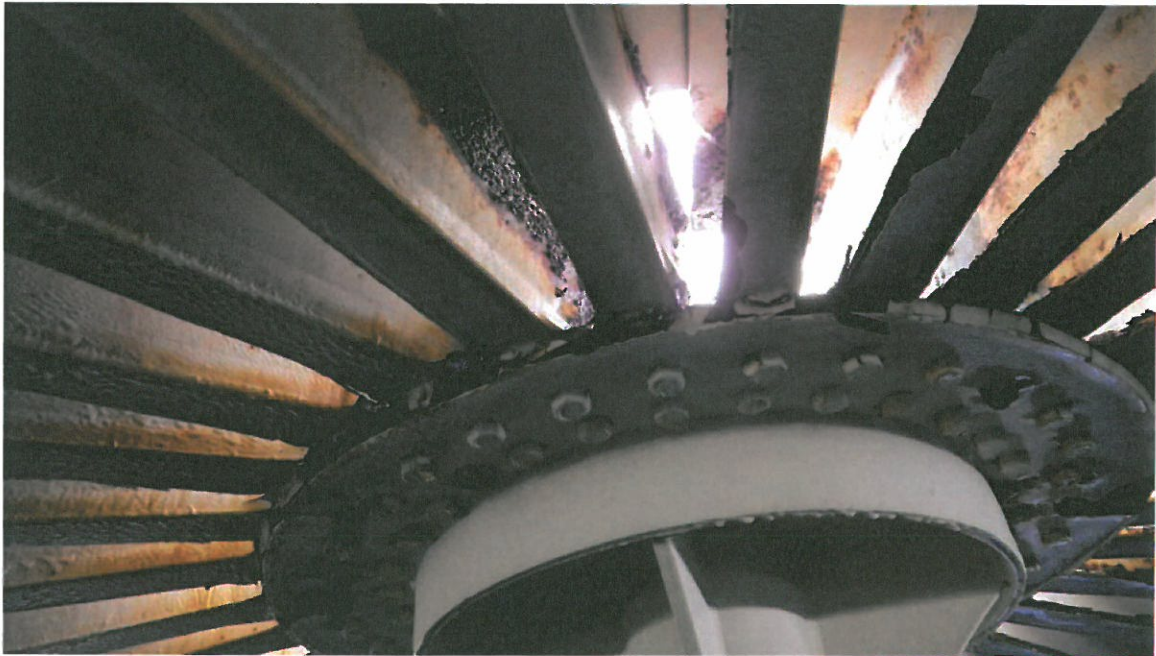
Photo 6 – Center Column Paint Failure & Corrosion
