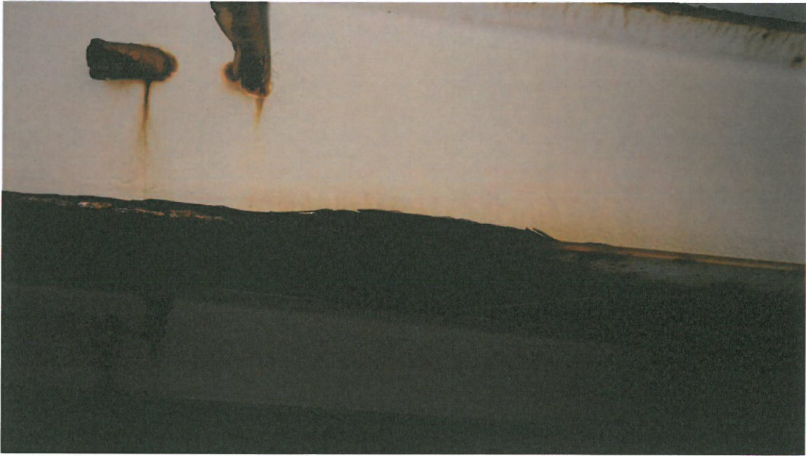
Photo 5 – Interior Channel Bottom Flange Corrosion
