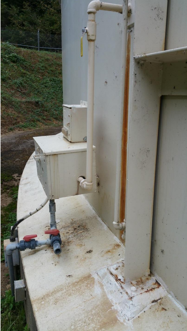
Photo 10: Sample Pump Enclosure (1 of 2)
