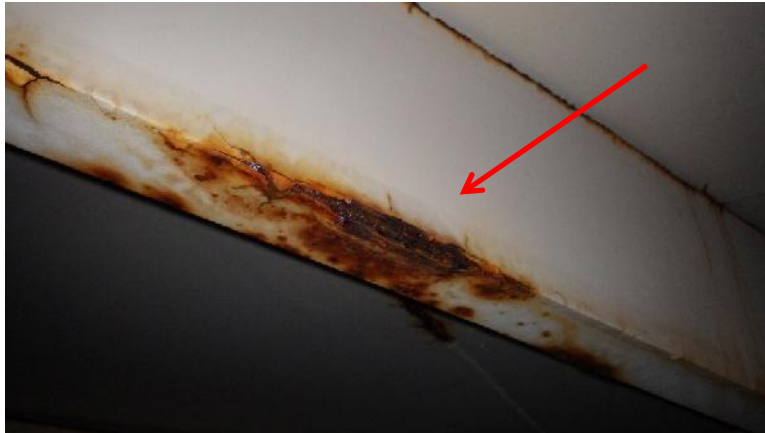
Photograph 1 – 1MG Reservoir interior – metal I-beam with paint (typ., indicated with red arrow) determined to contain lead and chromium.
