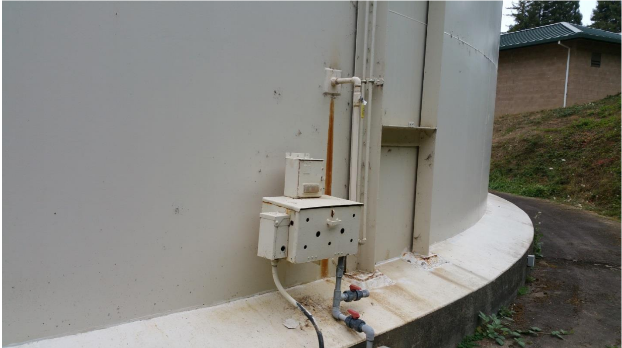
Photo 11: Sample Pump Enclosure (2 of 2)
