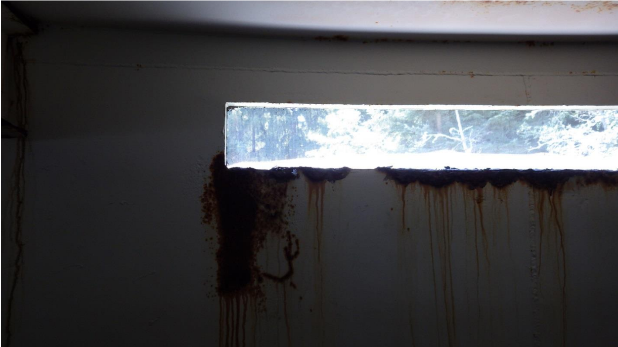
Photo 4: Typical Air Vent at Interior Side
