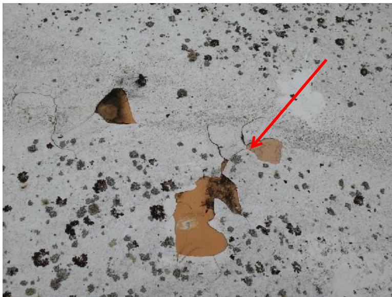
Photograph 2 – 1MG Reservoir exterior – detail view of metal roof with paint (typ., indicated with red arrow) determined to contain lead and chromium.
