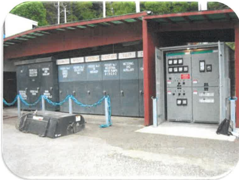
12kV Prior to Relocation Project
