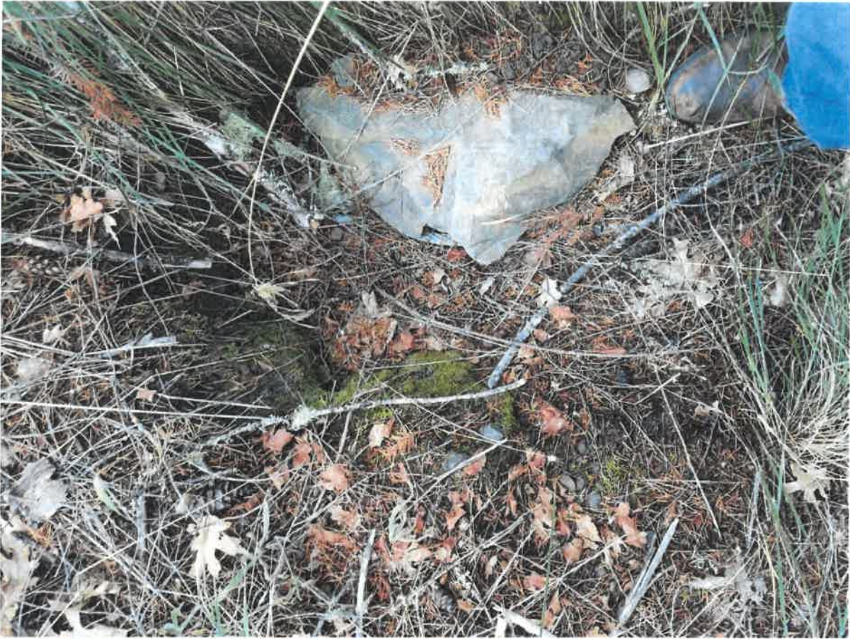
Photo 18-West End Anchor Deadman (buried under moss & vegetation)
