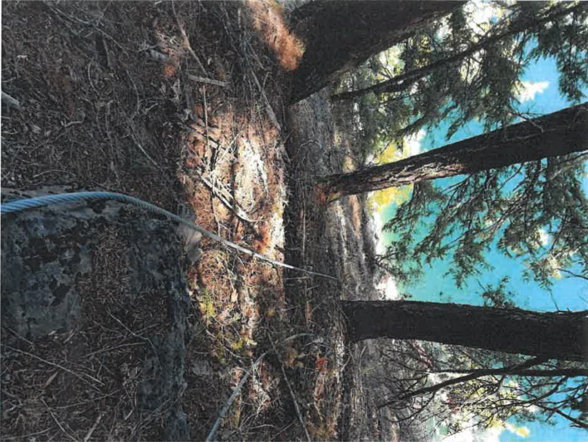
Photo 17-West End Anchor Cable (note rock but cable did not appear to be wearing on rock)
