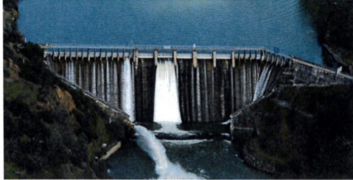
Scott Dam which is part of the Potter Valley Project. [Photo cropped by one from PG&E]
