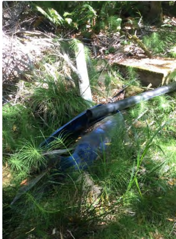
Ninety percent of waterflow being diverted from waterway.
