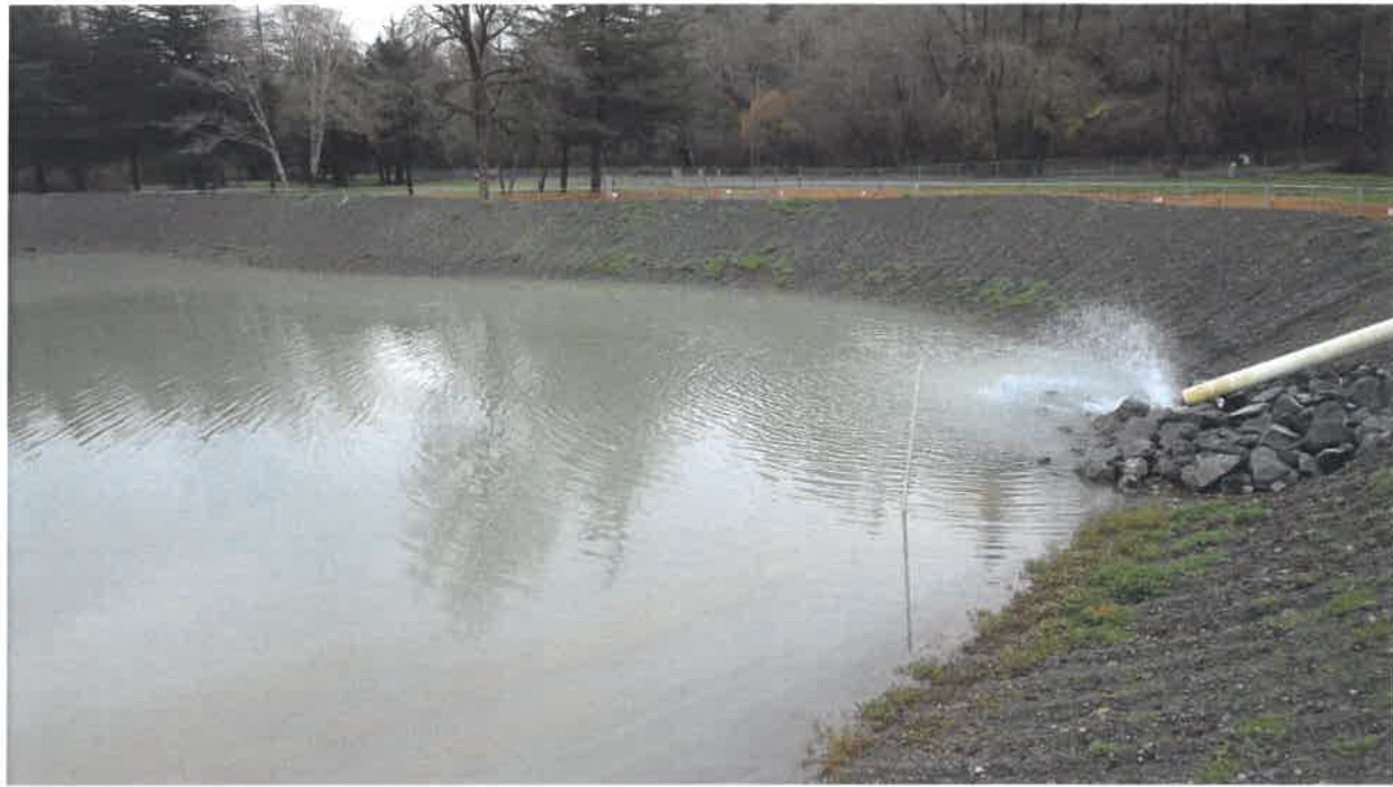
Figure 6: Percolation pond; used to settle water pumped out of the collectors during construction
