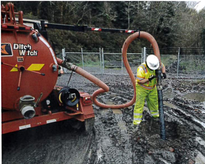
Boom deployed during operation, notice how it supports the vacuum line above the operator.
