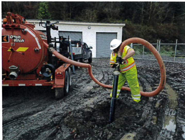
Boom not deployed, notice all the weight of the suction line is on the operator's shoulders.
