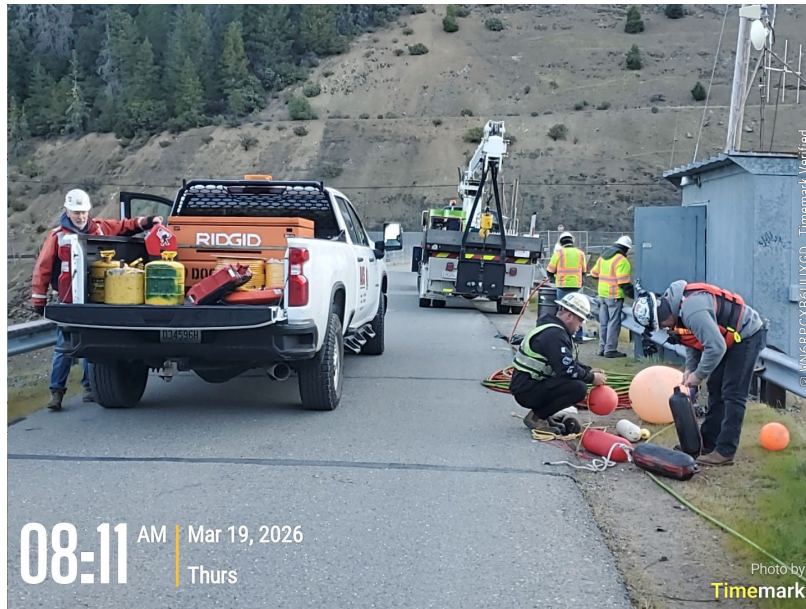
AUS dive crew and District staff preparing equipment on the dam crest, March 19, 2026.
