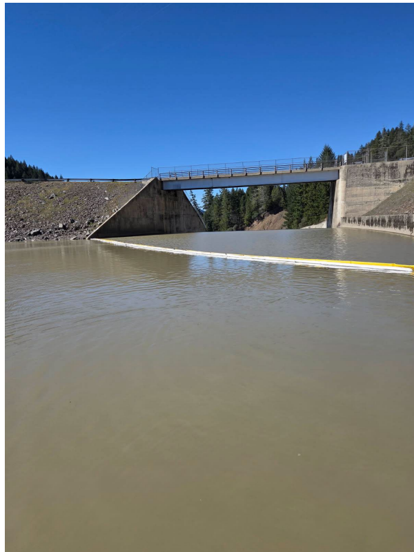
Containment boom deployed between the spillway walls at R.W. Matthews Dam.
