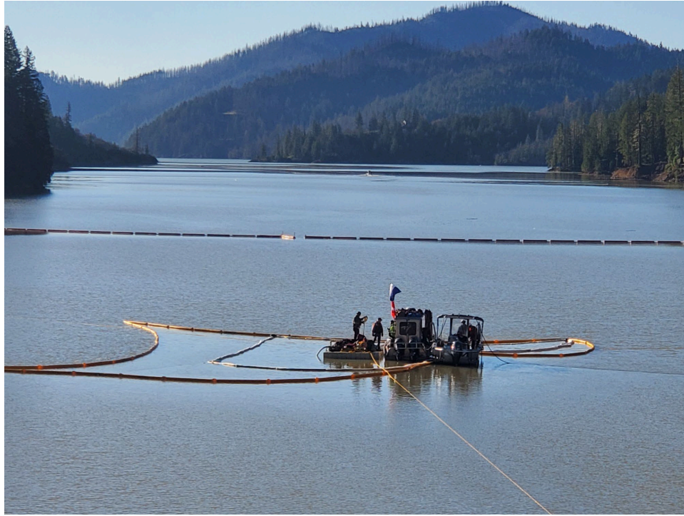
AUS dive vessel positioned over the intake structure within oil containment boom, Ruth Lake.
