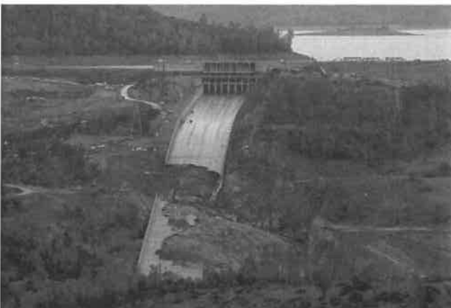
The Oroville Dam's damaged spillway in 2017. Justin Sullivan/Getty Images
